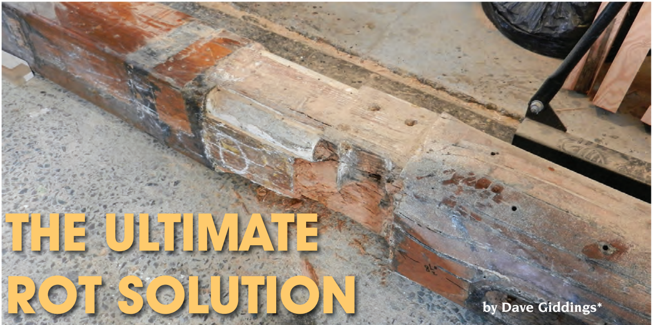
Figure 1 – The damaged section of mast.
