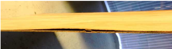
Figure 3 – Cut Plywood showing Delamination Issues
